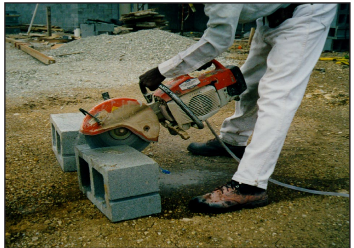
Handheld masonry saw using water for dust control while cutting cinder blocks. (Photo courtesy of New Jersey Department of Health).
