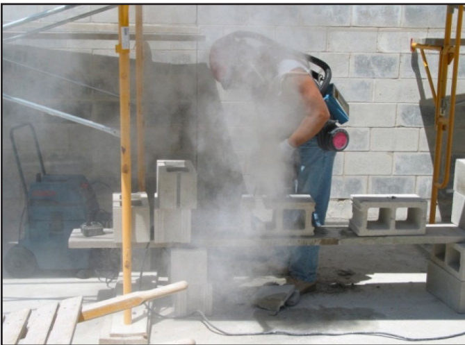
Handheld masonry saw without dust controls creates silica dust while cutting cinder blocks. (Photo courtesy of New Jersey Department of Health).
